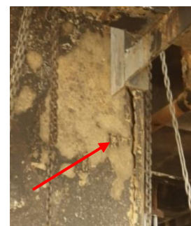
Figure 7. Crack at column E1.
