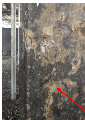
Figure 6. Crack at column A2.
