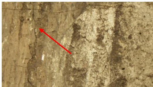
Figure 5. Spalling and crack at column E2.
