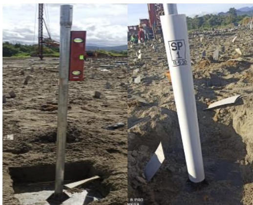
Figure 3. Installed instrumentations at site.
