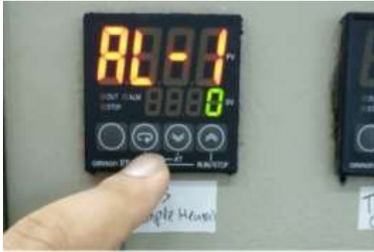
Figure 7. Operation of Temperature Controller in Methanol Testplant
