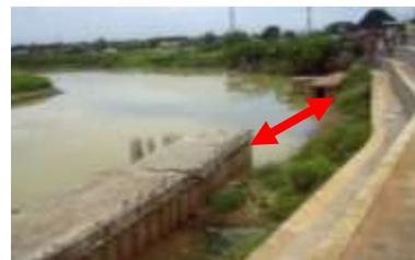
Figure 9. A Collapsed Structure at the Middle Section
