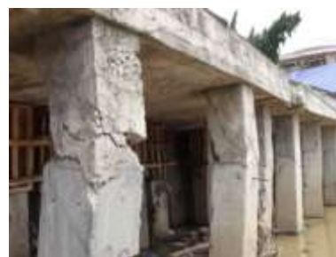
Figure 10. Broken Pile at Joint
