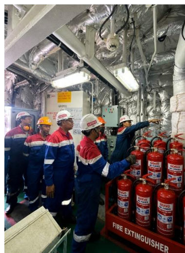
Figure 5. Fire Extinguisher Station Review by Crew Members Source: Field observation (2025)
