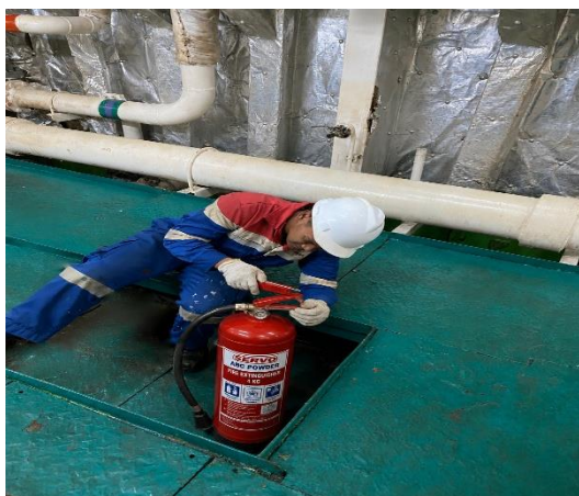
Figure 4. Development and Inspection of Portable Fire Extinguishers Source: Field observation (2025)
