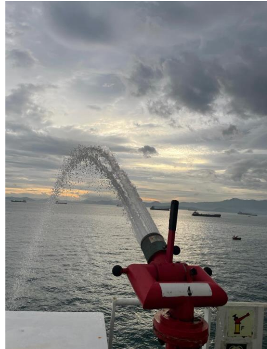
Figure 7. Deck Fire Monitor Source: Field observation (2025)
