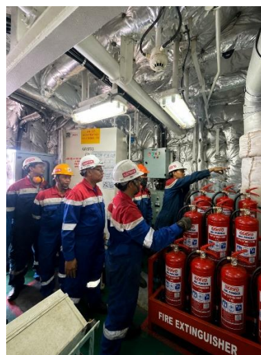
Figure 5. Fire Extinguisher Station Review by Crew Members
